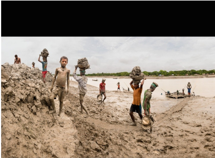
Building Up The Embankment Along Kholpetua River, 21 minutes 30 seconds Workers dredge the river channel, lowering the bottom of the river while building up the embankments to create a topography where gravity pulls water away from villages and fields.
